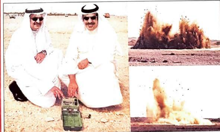
■ Bahrain blasted its way into the future yesterday with the start of excavation work on a project which will bring Formula One motor racing to the country. Experts will be clearing 500,000 cubic metres of rock to build the Bahrain Racing Circuit in Sakhir. The first two explosions were staged between noon and 1pm, at the 300 hectare site. F1 work begins - Page 11
